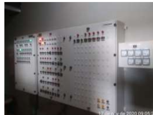
Painel de Controle
